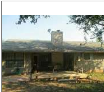
Service Drop and tree branches needing to be trimmed
