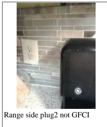
Rangeside kitchen plug not GFCI
