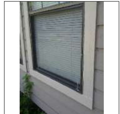
Exterior window pane missing from double paned window on front bedroom
