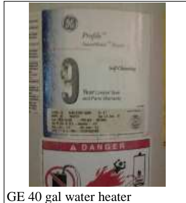
GE 40 gal water heater
