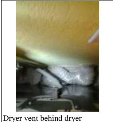
Dryer vent behind dryer
