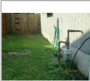
Negative grading towards northside foundation, lack of swale
