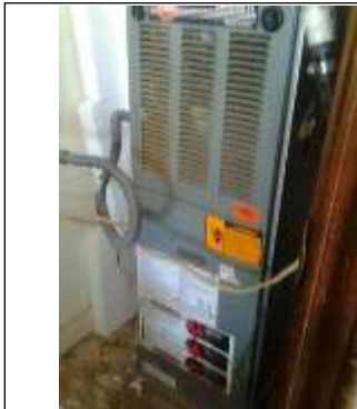
Furnace cabinet gas line not bonded
