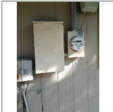
220-volt service meter
