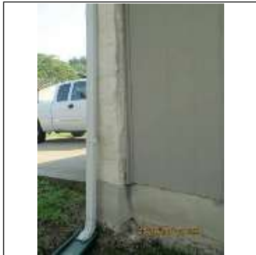
Damaged downspout, erosion of soil, and deterioration of foundation.
