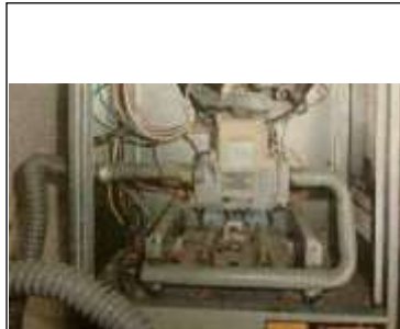
Flexline coming into furnace
