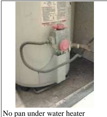
No pan under water heater
