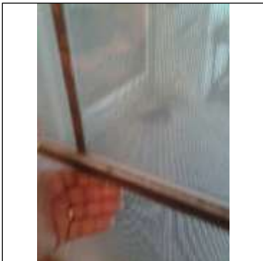
Dining room window springs do not hold window in an open position.
