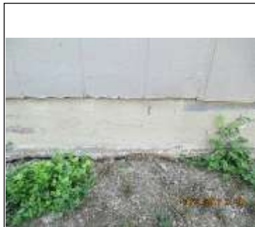
Shows erosion of soil away from foundation
