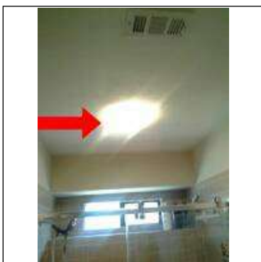
Vent light unit in bathroom
