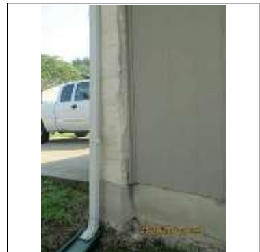
Deteriation of foundation from erosion
