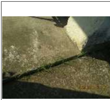
Transition between front porch and sidewalk has settled and needs to be sealed
