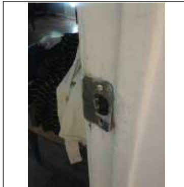
Damaged master bedroom door hardware
