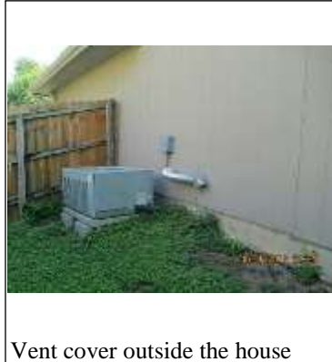
Vent cover outside the house
