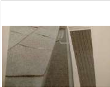
Roof material in gutter, another sign of normal wear and gutter needs cleaning
