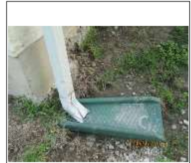
Another shot of damaged downspout
