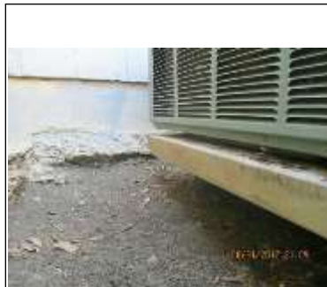
Erosion of soil at the foundation on westside.
