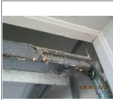
Garage door weather stripping is torn
