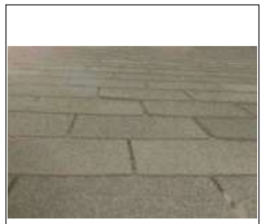
Some evidence of wear and shingles standing or pulled up.
